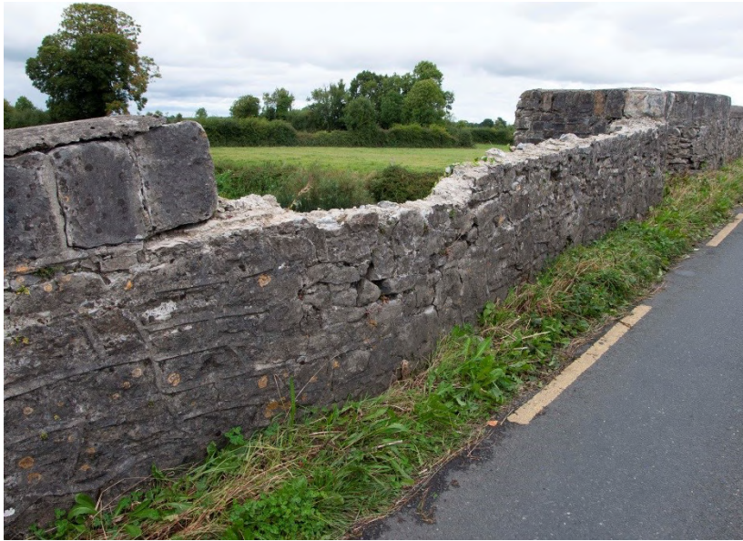
Plate 26: Detail of recent damage to north approach wall on west side of bridge
