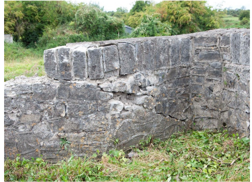
Plate 27: Cracking visible in triangular cut-water in north wall on west side of bridge
