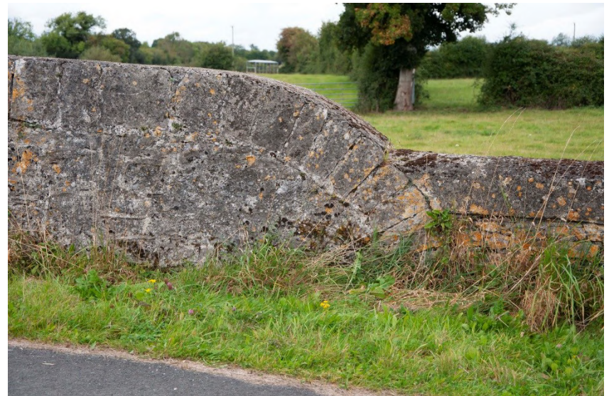
Plate 29: Detail of masonry in north approach wall on east side of bridge
