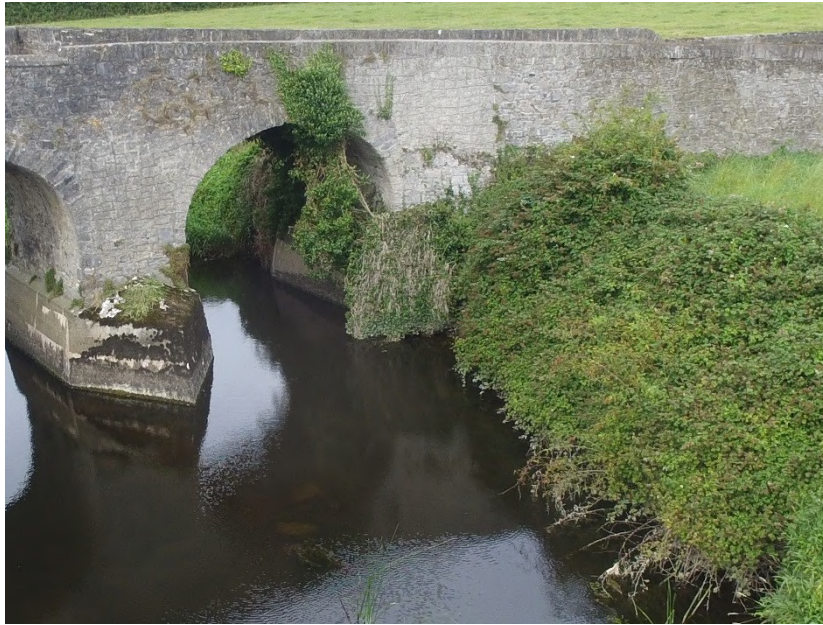
Plate 22: Detail of abutment and side wall on east side of south-facing elevation
