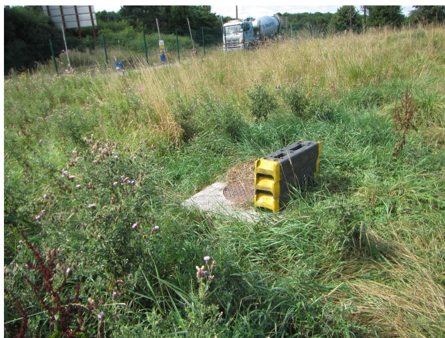
Plate 18 Manhole within the triangular field.
