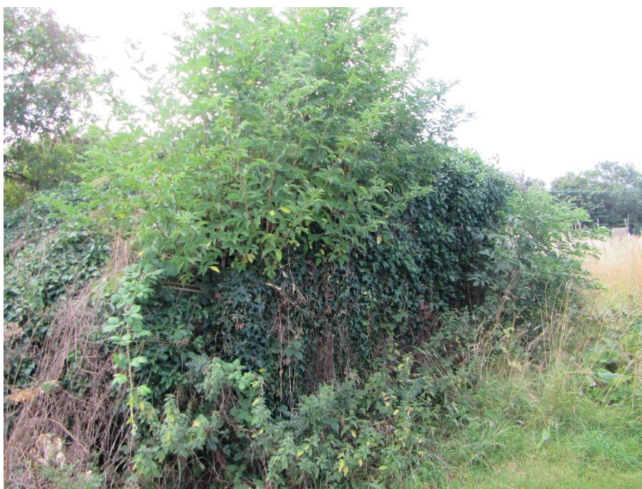
Plate 17 Overgrown wall at the southeast of the laneway.
