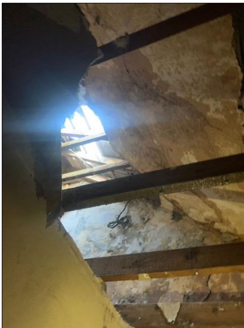
Plate 3.4 – Source of draught into the dwelling house.
