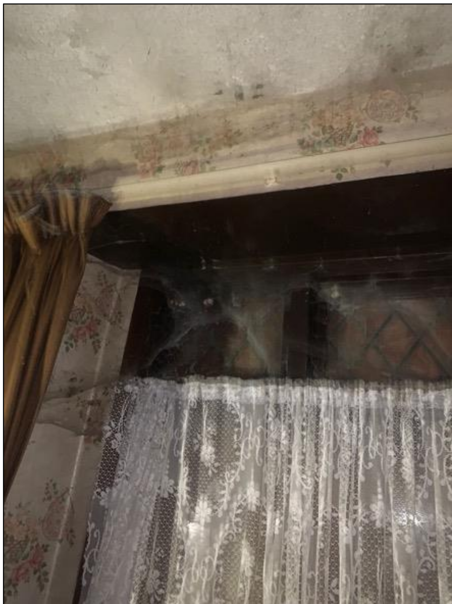
Plate 3.3 – Cobwebs present in existing house.
