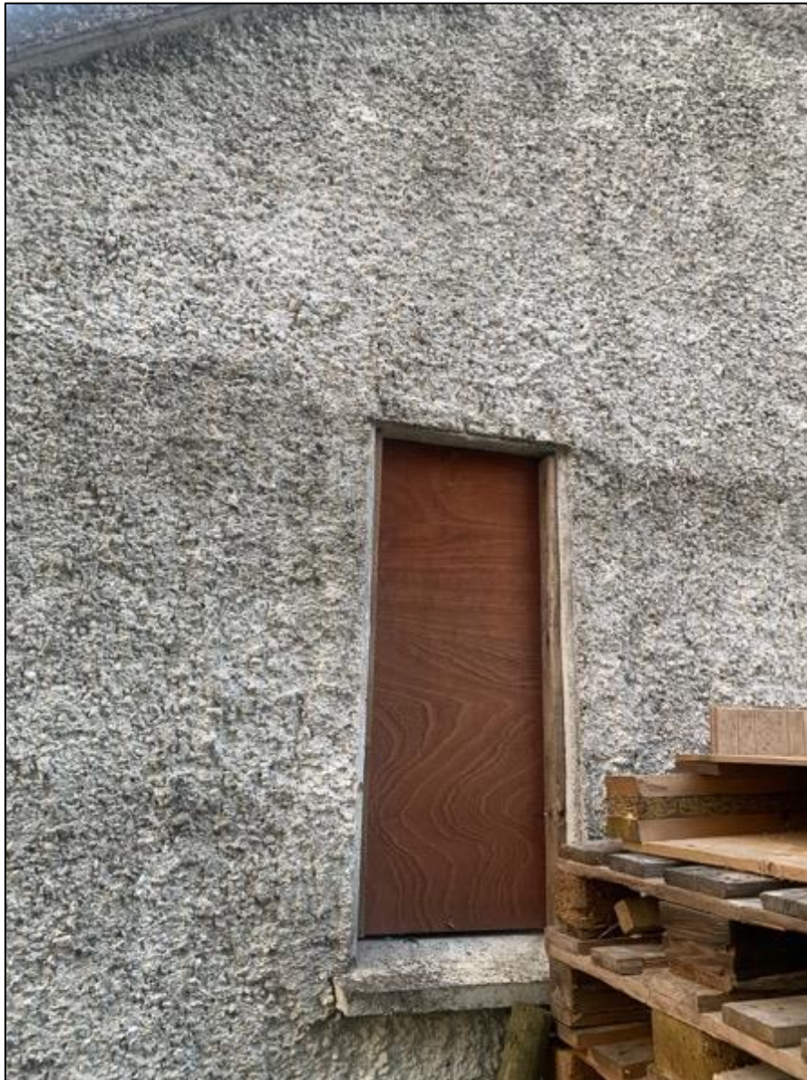
Plate 3.2 – Boarded windows in existing dwelling house.
