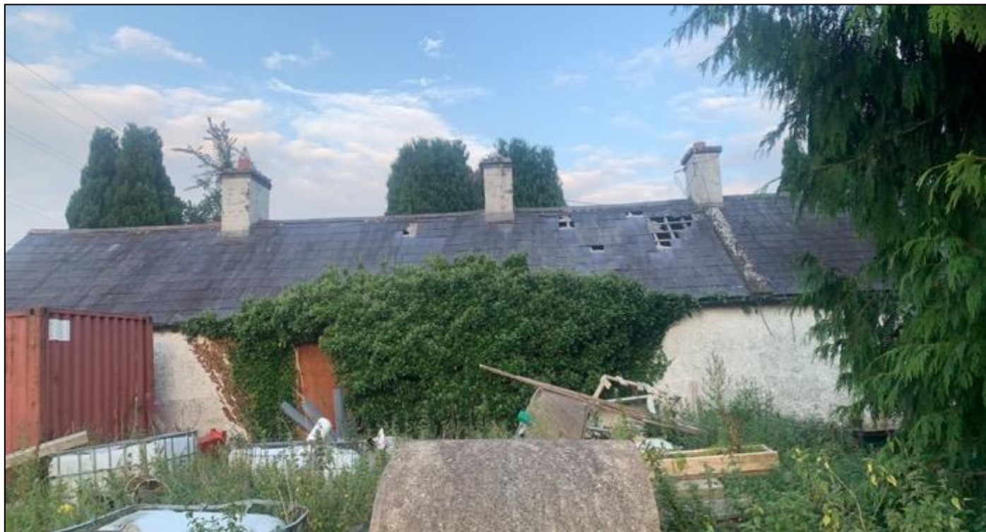
Plate 3.1 – Partial collapsed section of roof of existing house.
