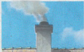
Chimneys are a risk if not cleaned
