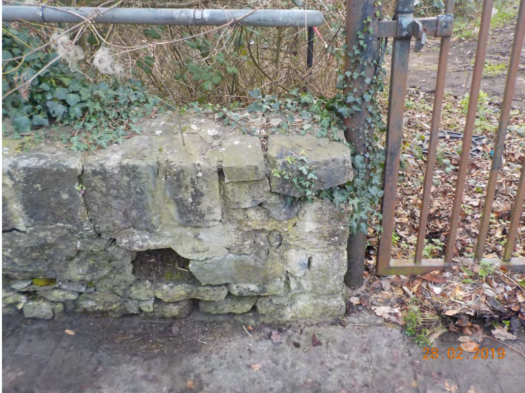
Photograph 3-25: Wall to be Raked and Repointed
