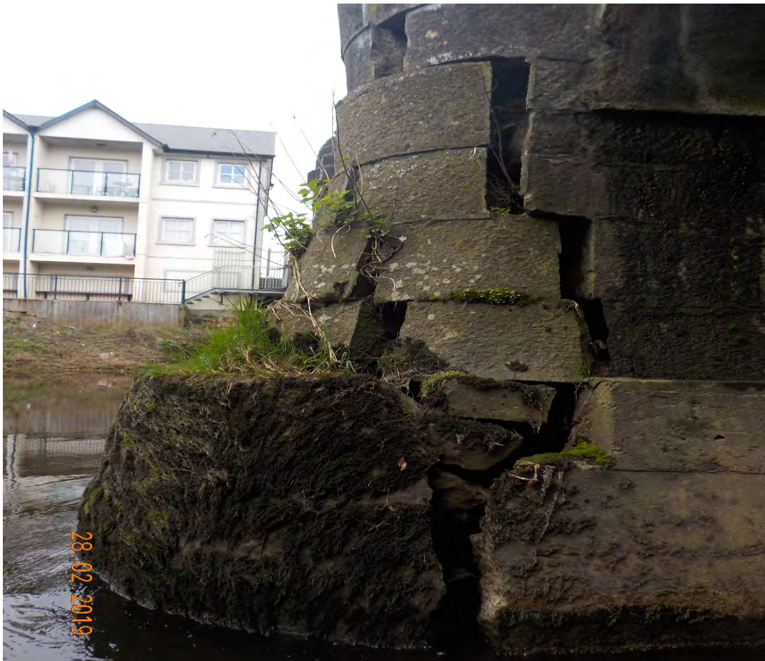
Photograph 3-54: Pier 2 – Settling away from Bridge
