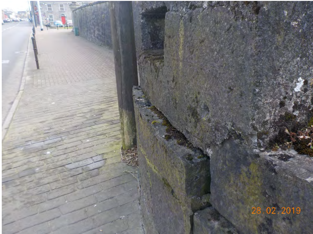
Photograph 3-13: Settlement of Bunker on Downstream side
