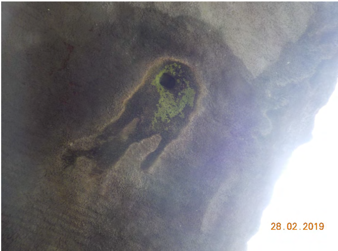
Photograph 3-56: Hole in Upstream and Downstream of Bridge Deck 2
