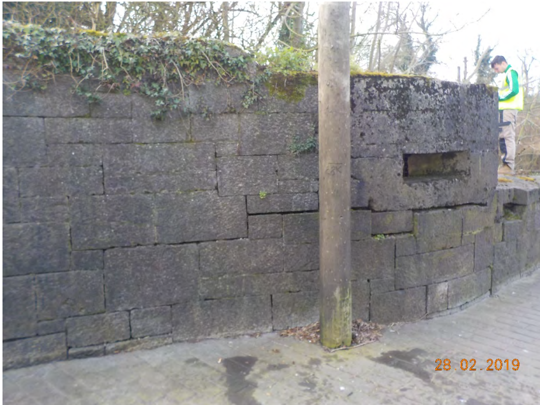
Photograph 3-15: Overall View of Bunker Settlement
