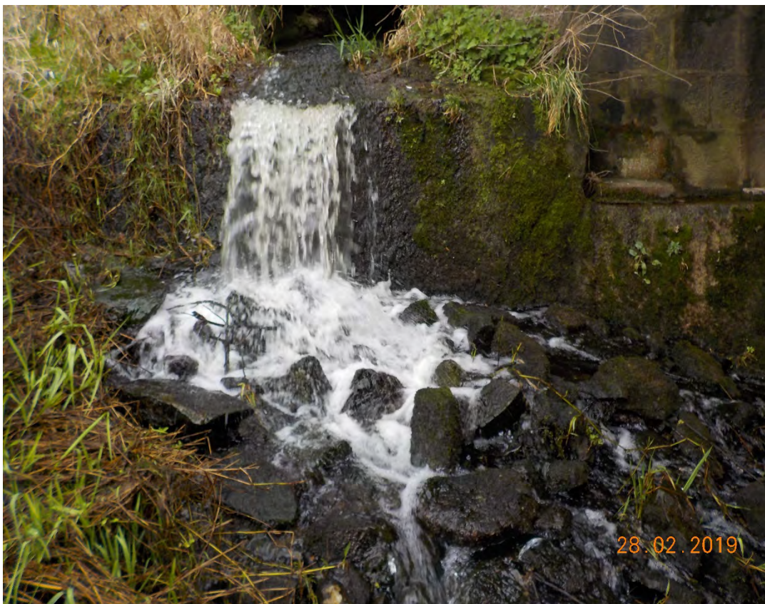
Photograph 3-48: Culvert on Upstream Embankment Failing
