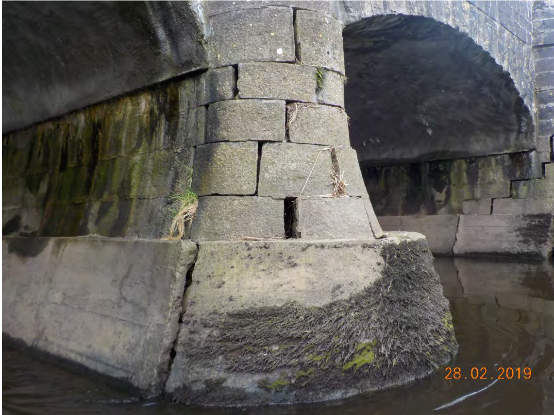
Photograph 3-68: Pier 3 – Natural Scouring
