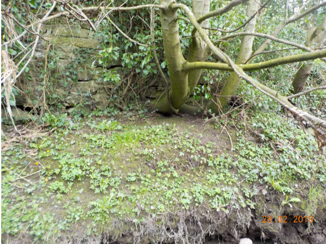
Photograph 3-39: Tree's to be removed on Downstream Left Embankment
