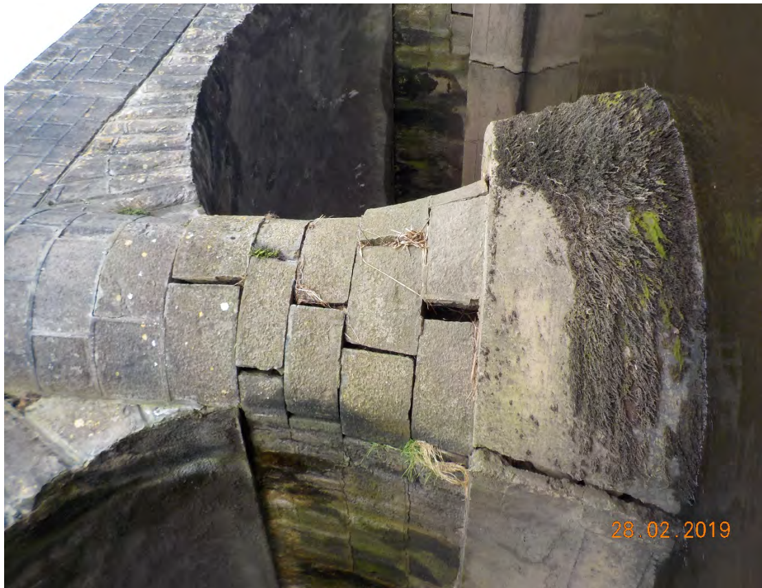
Photograph 3-66: Pier 3 – Natural Scouring
