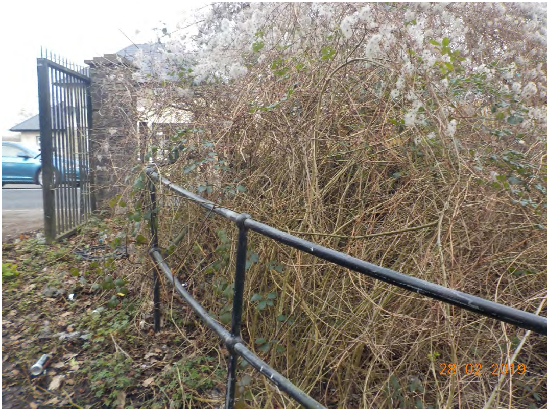
Photograph 3-42: Overgrown Vegetation on Downstream Right Embankment
