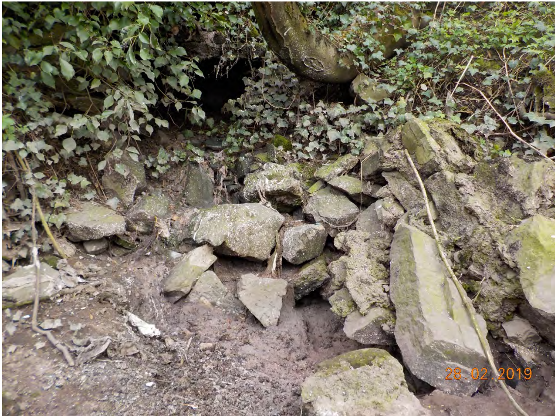
Photograph 3-78: Outfall to be reconstructed
