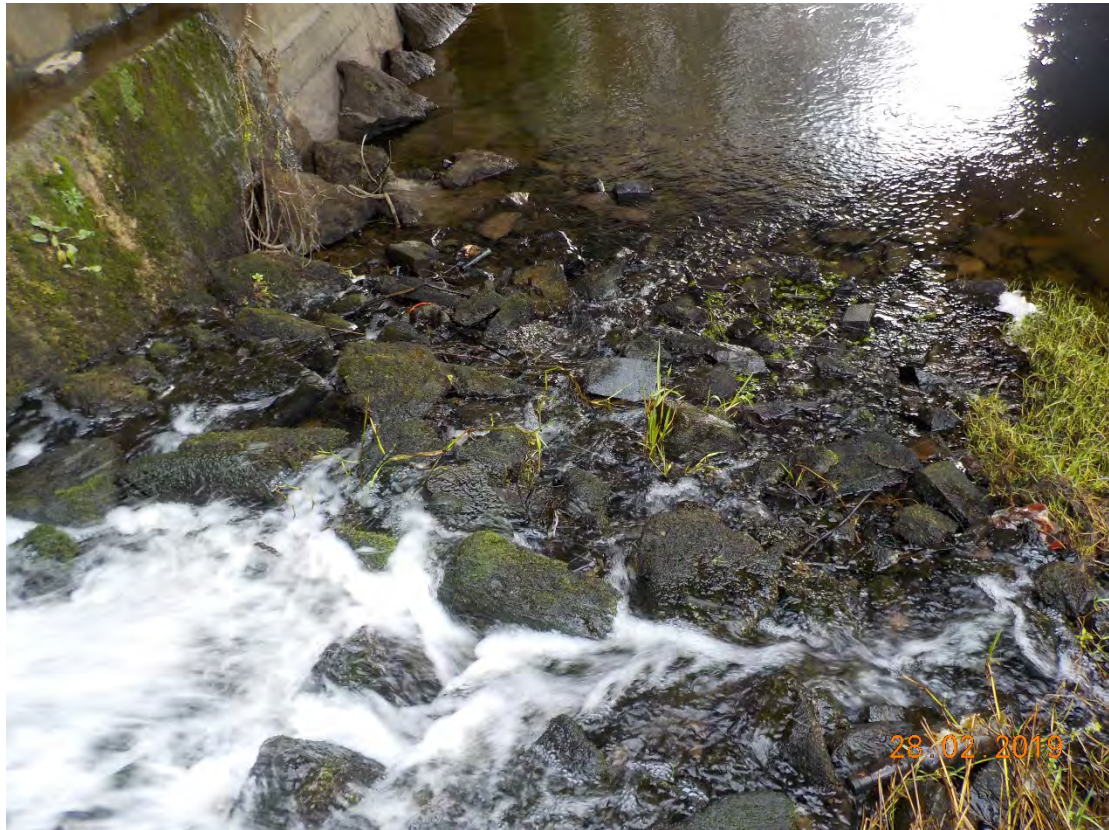
Photograph 3-49: Culvert on Upstream Embankment Failing
