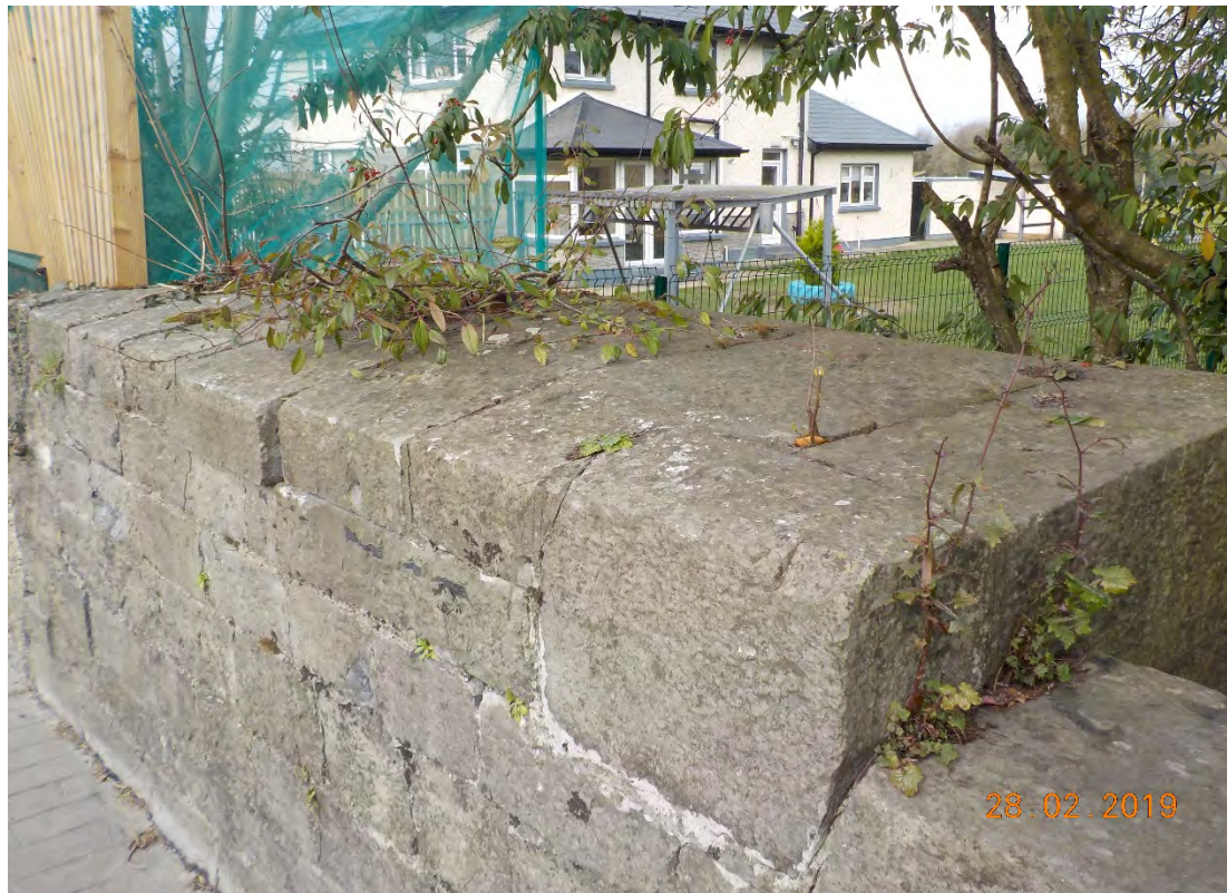
Photograph 3-28: Tree Roots in Capping on Upstream Parapet
