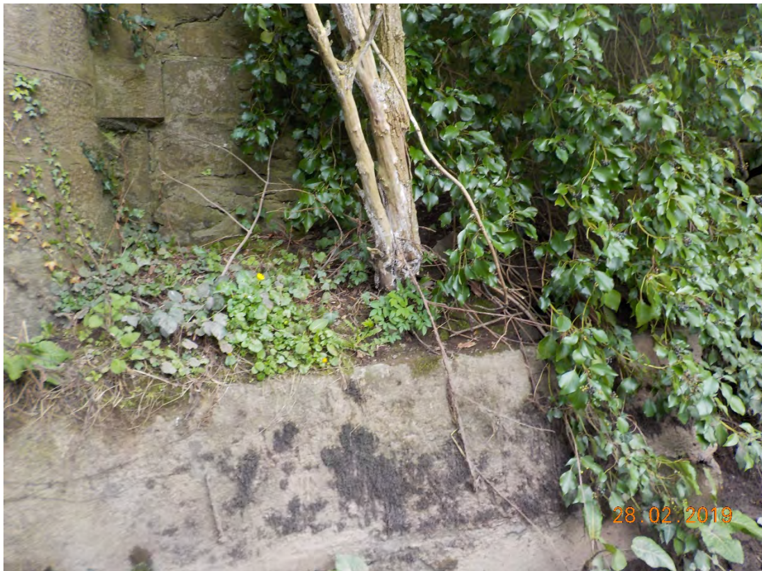
Photograph 3-40: Tree's to be removed on Downstream Left Embankment
