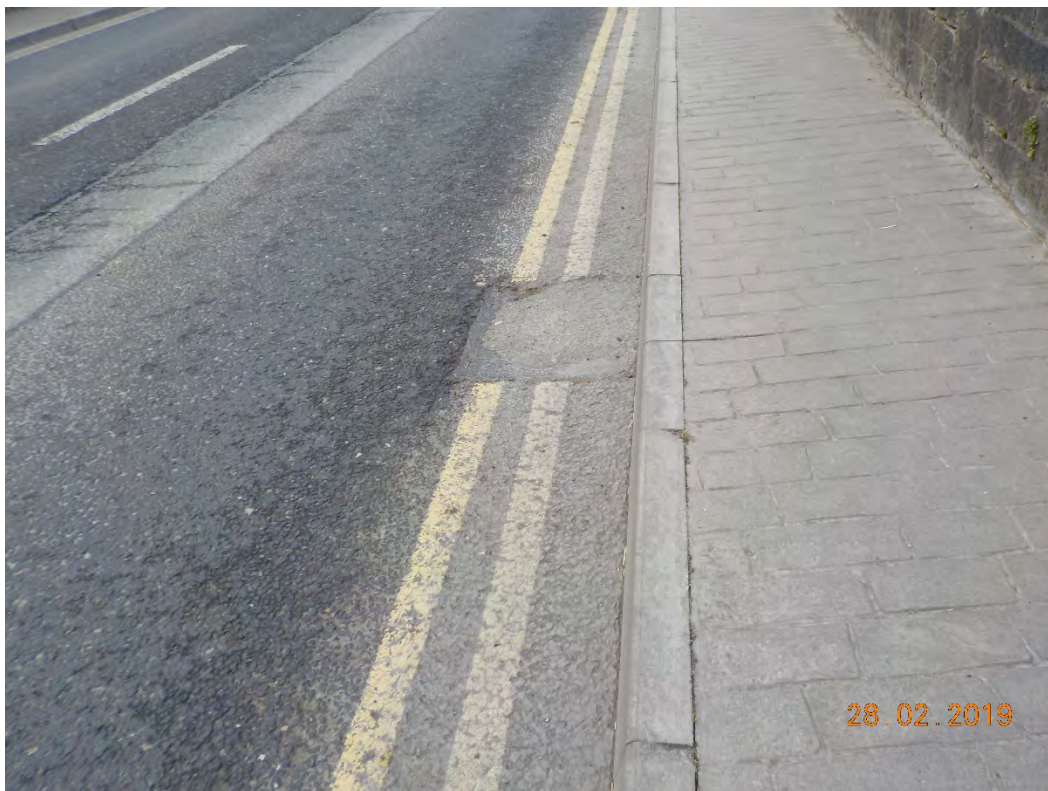
Photograph 3-2: Poor Patch Repair on Bridge Surface
