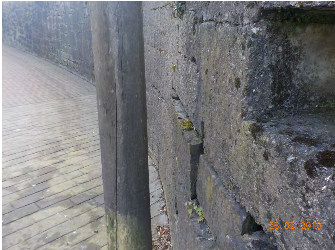
Photograph 3-14: Settlement of Bunker on Downstream side
