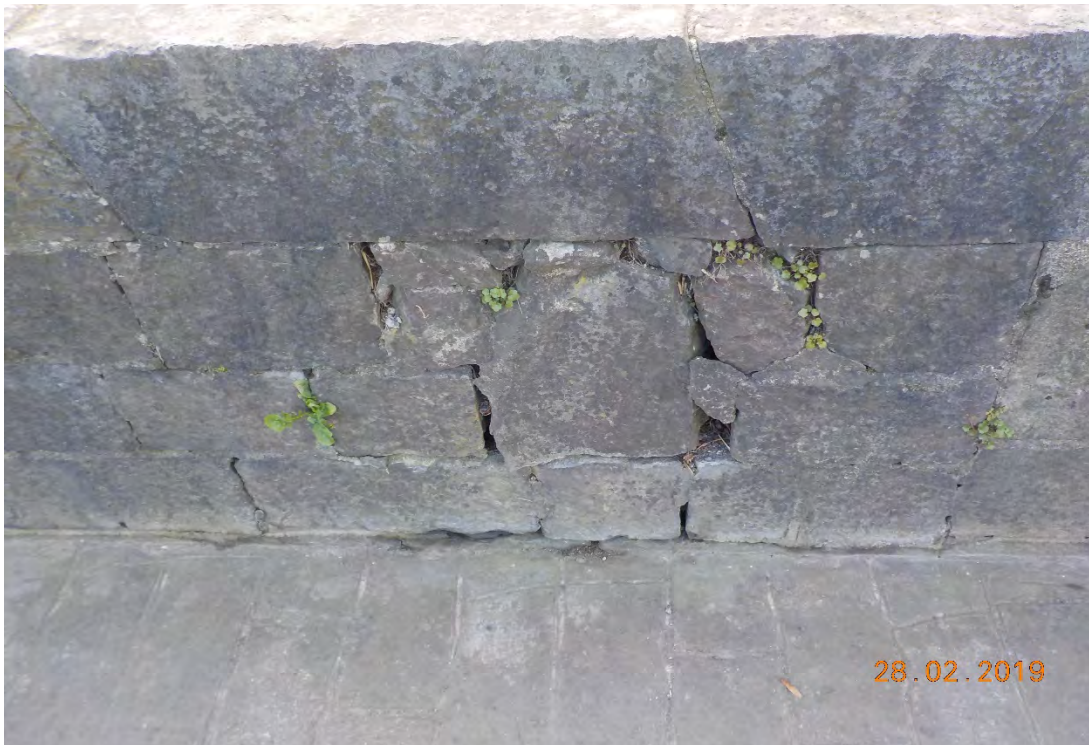
Photograph 3-19: Masonry Dislodged on Downstream Roadside Parapet
