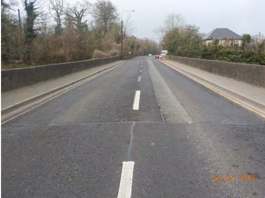
Photograph 3-3: Poor Patch Repair on Bridge Surface
