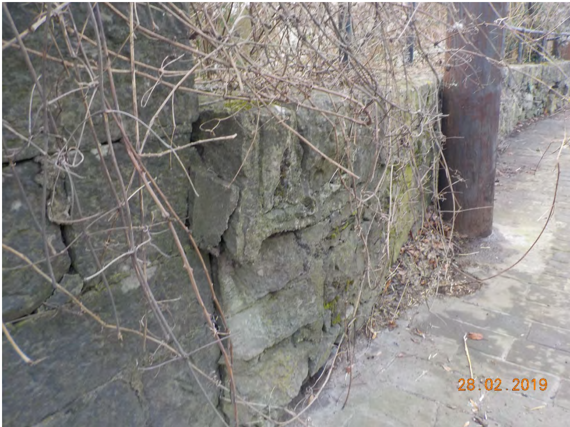
Photograph 3-22: Capping to be reset on Downstream Parapet
