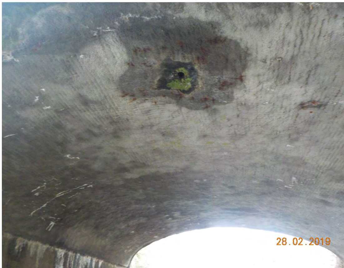
Photograph 3-52: Arch 1 - Hole in Upstream Bridge Deck
