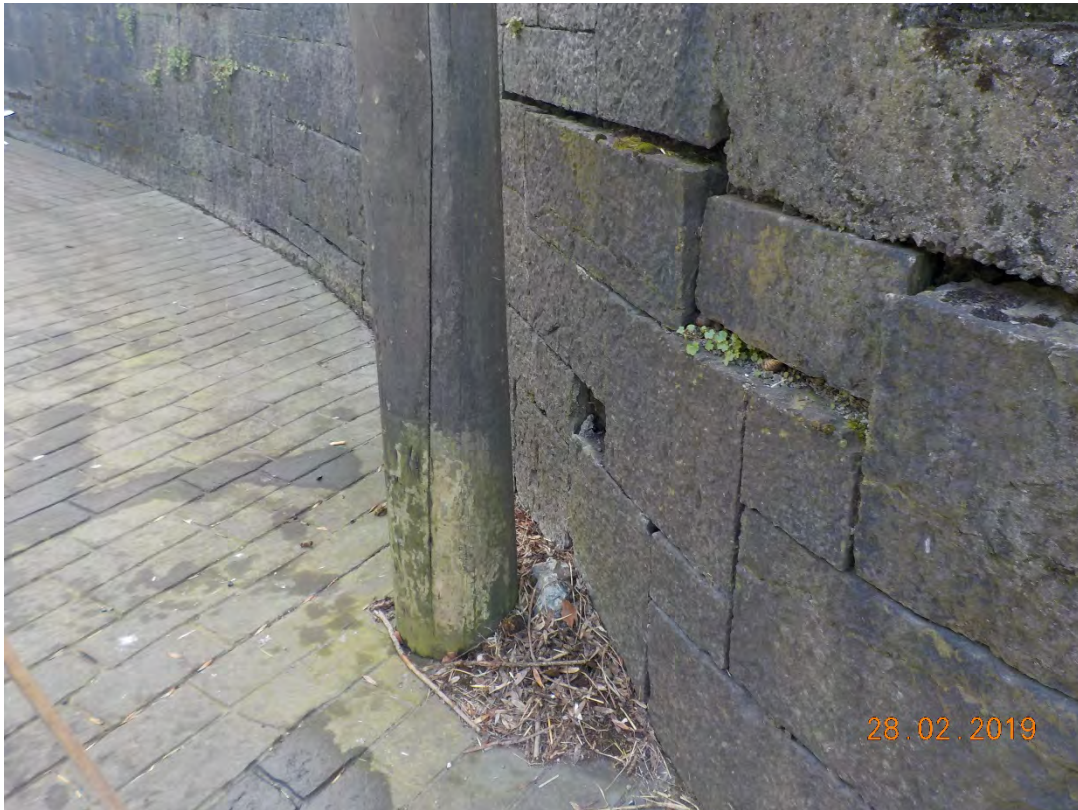
Photograph 3-11: Missing Masonry on Downstream Roadside Parapet
