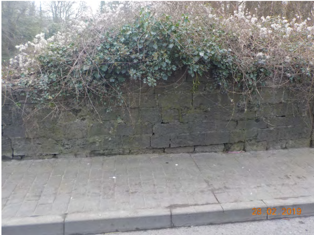
Photograph 3-21: Bulging on Section of Downstream Parapet Wall
