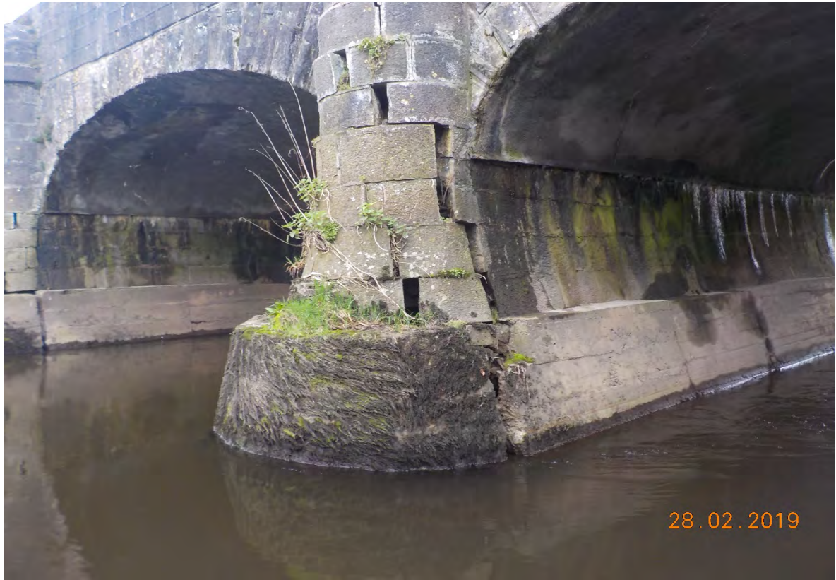
Photograph 3-55: Pier 2 – Settling away from Bridge
