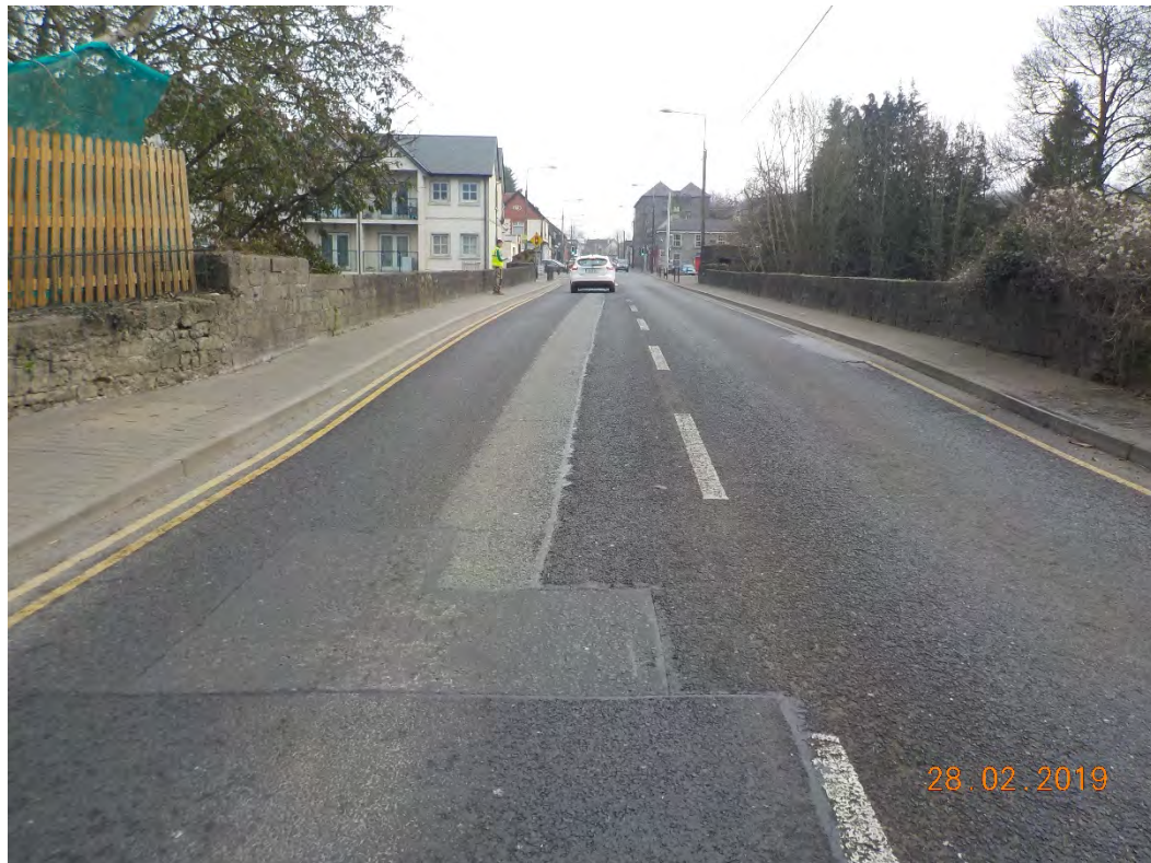
Photograph 3-4: Poor Patch Repair on Bridge Surface
