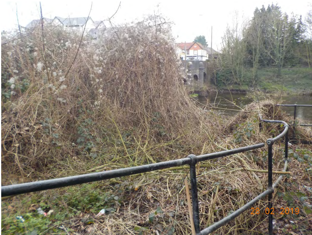
Photograph 3-41: Overgrown Vegetation on Downstream Right Embankment
