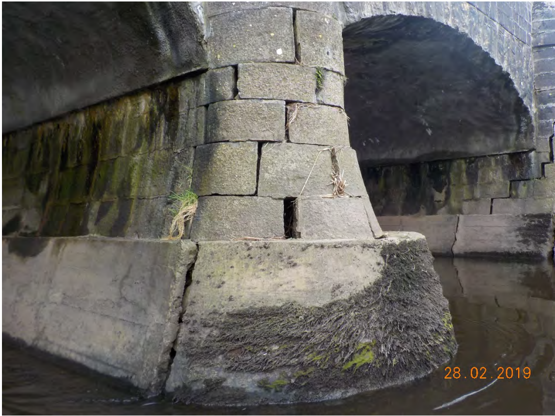
Photograph 3-67: Pier 3 – Natural Scouring
