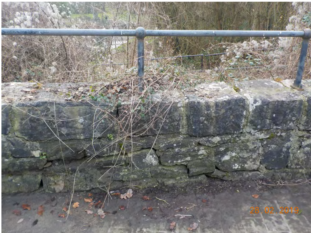
Photograph 3-24: Wall to be Raked and Repointed
