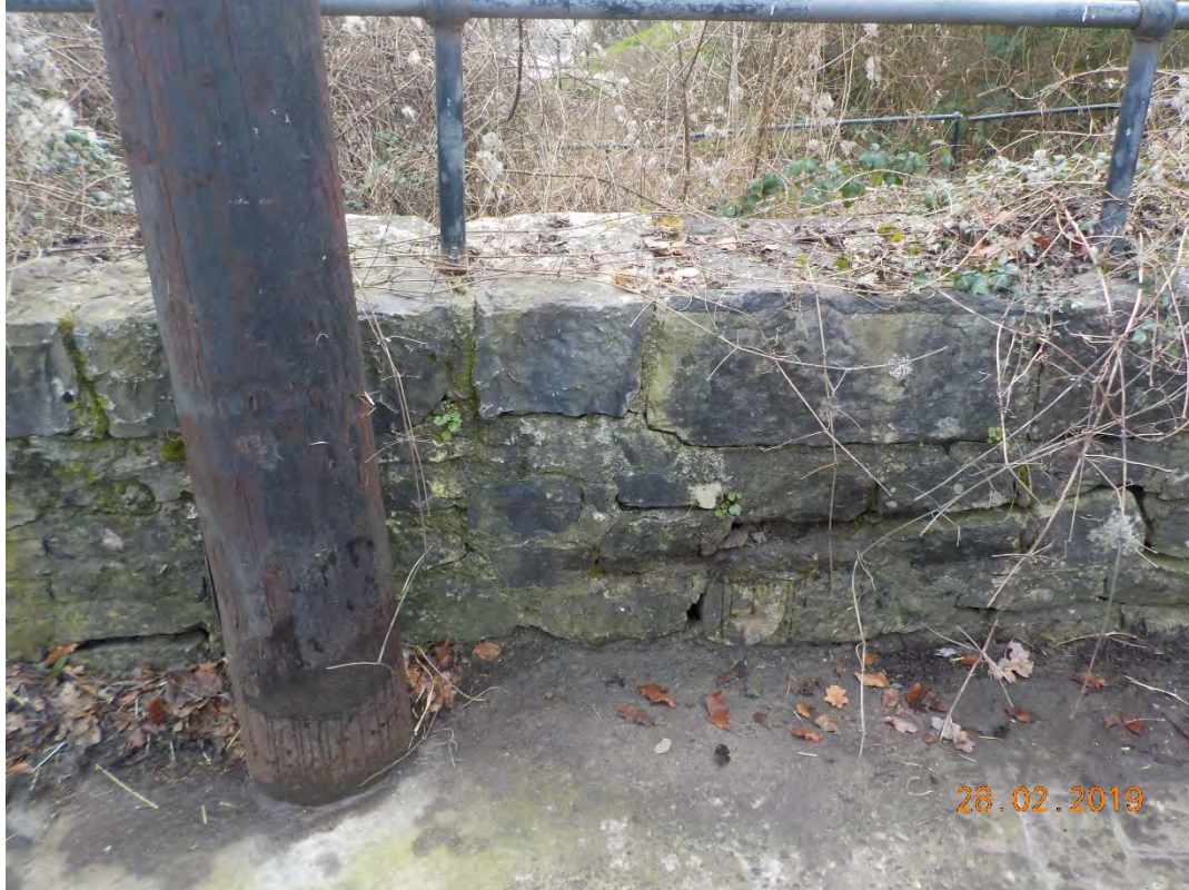
Photograph 3-23: Wall to be Raked and Repointed
