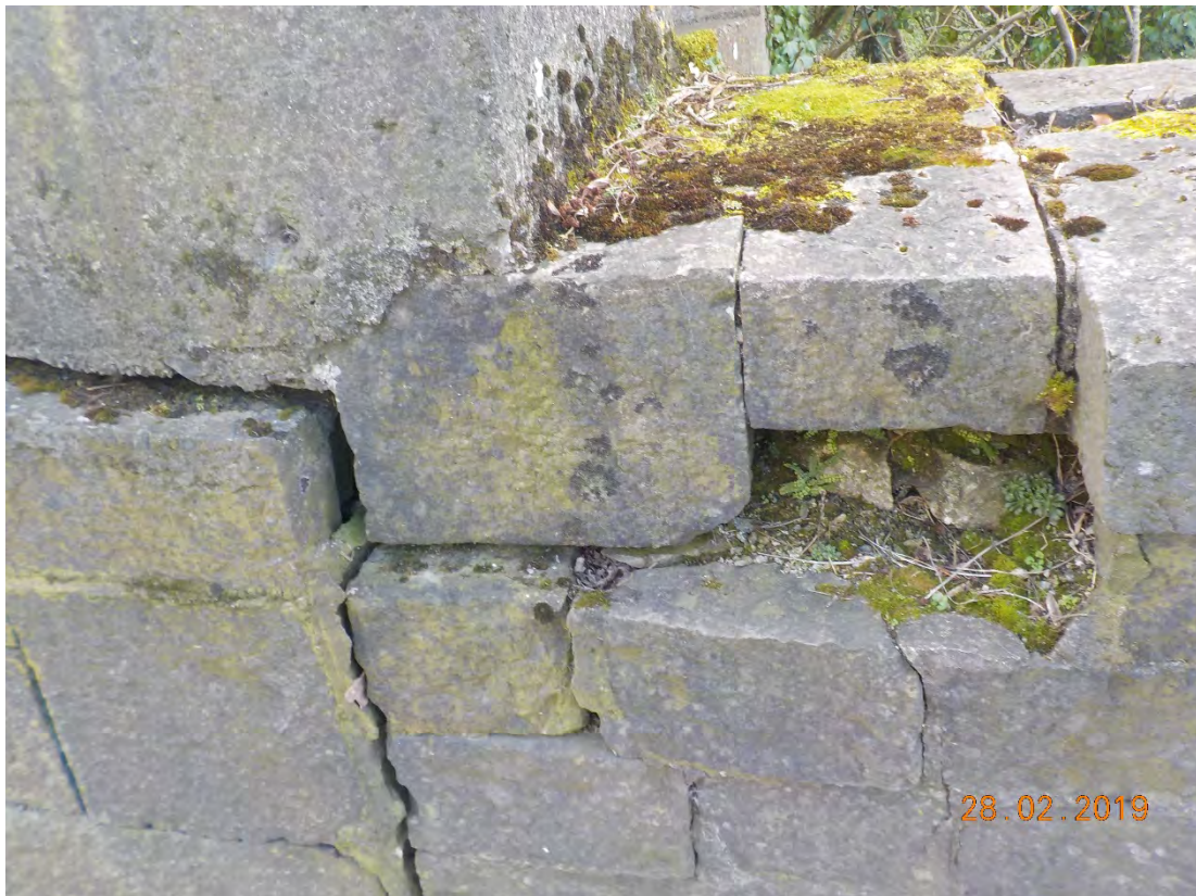
Photograph 3-12: Settlement of Bunker on Downstream side
