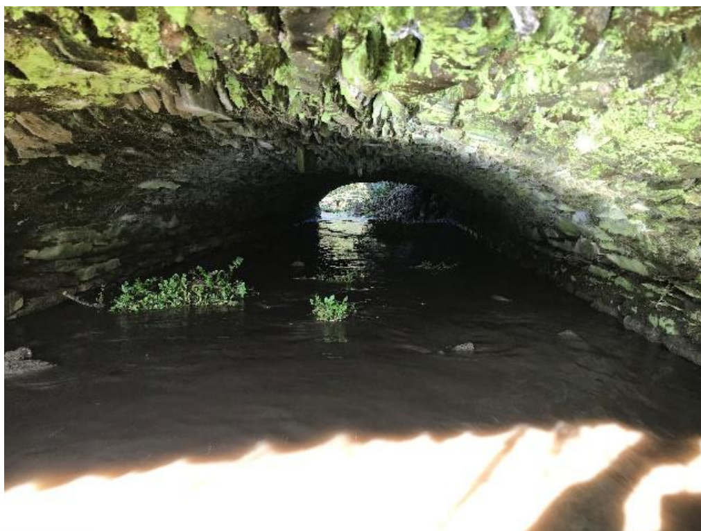
Figure 3: Loss of mortar in joints and vegetation growth
