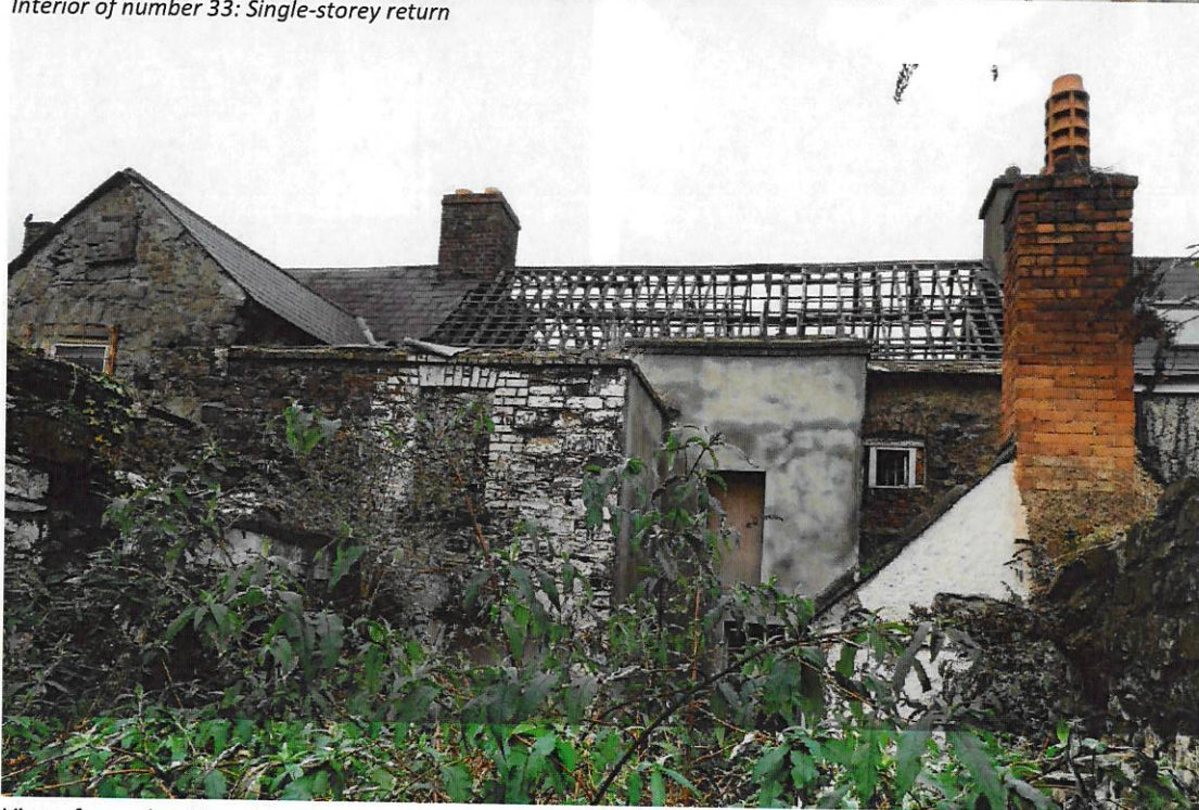
View of rear elevation of number 33, two-storey return (left), projecting central bay and single-storey return (right)
