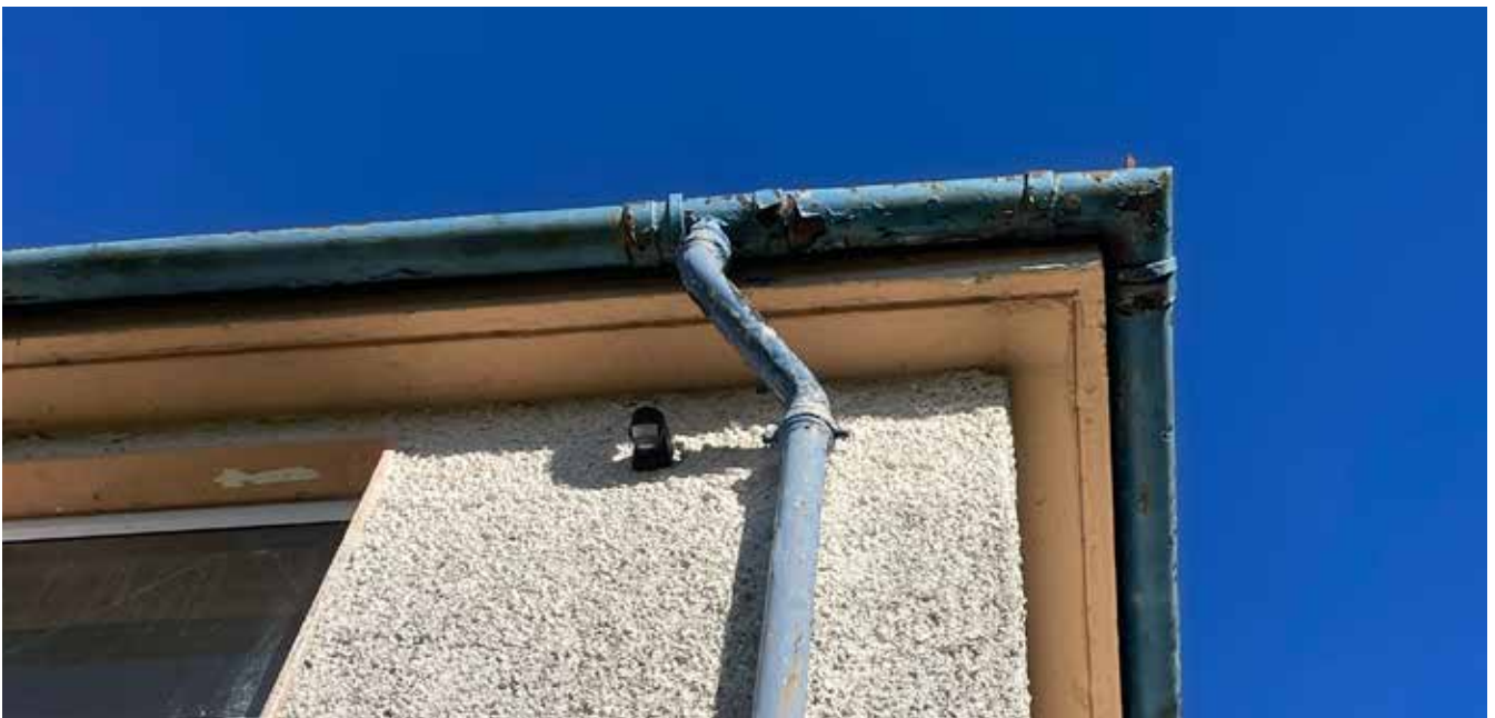
Fig.02 - Original cast rainwater goods, sections in need of repair.
