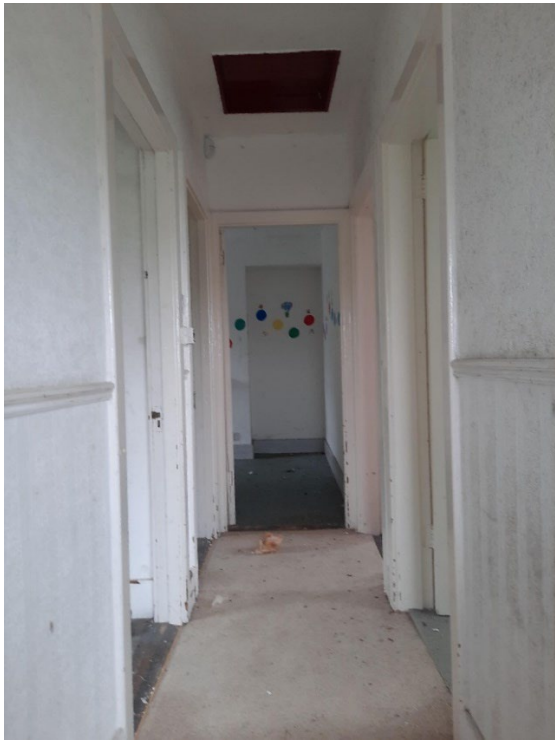
Photo G13 – First floor landing
