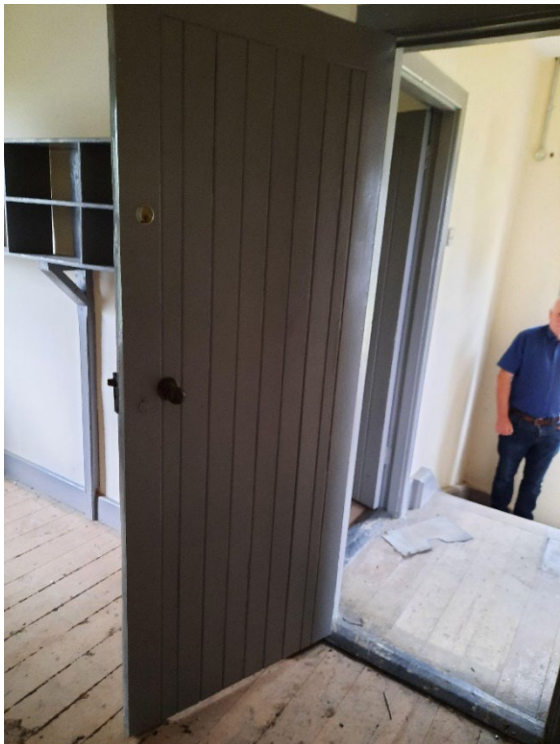
Photo G28 – First floor Landing
