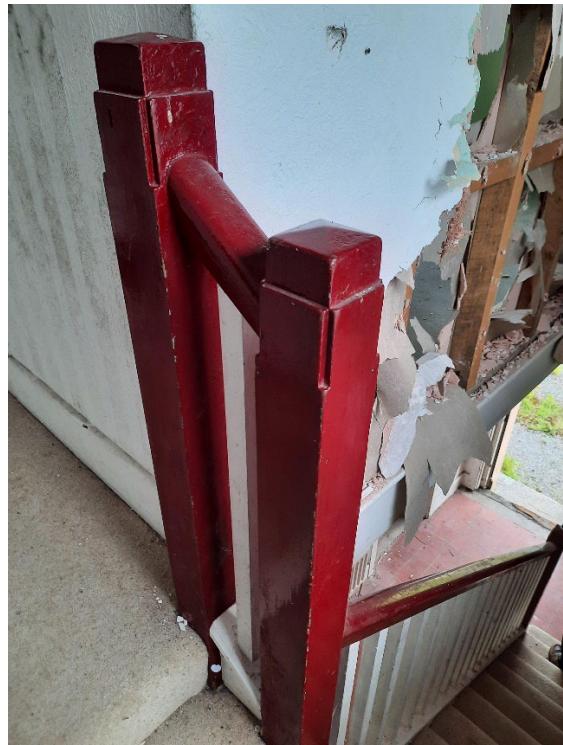
Photo G14 – First floor landing
