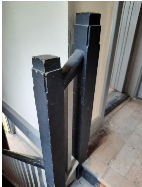
Photo G29 – First floor Landing
