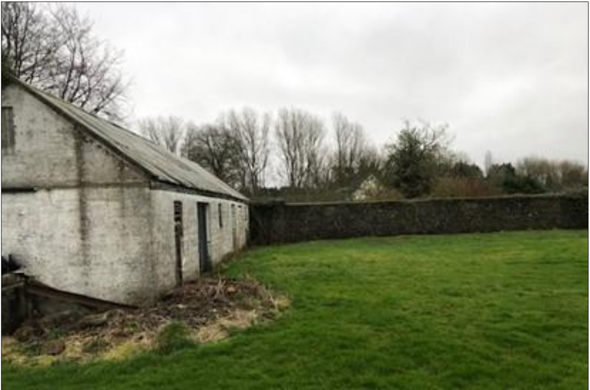
Plate 21: View south of the outbuilding and rear wall of the convent garden. The outbuilding is a late addition (it does not appear on the first or last edition of the 1:10,560 OS map for the town).
