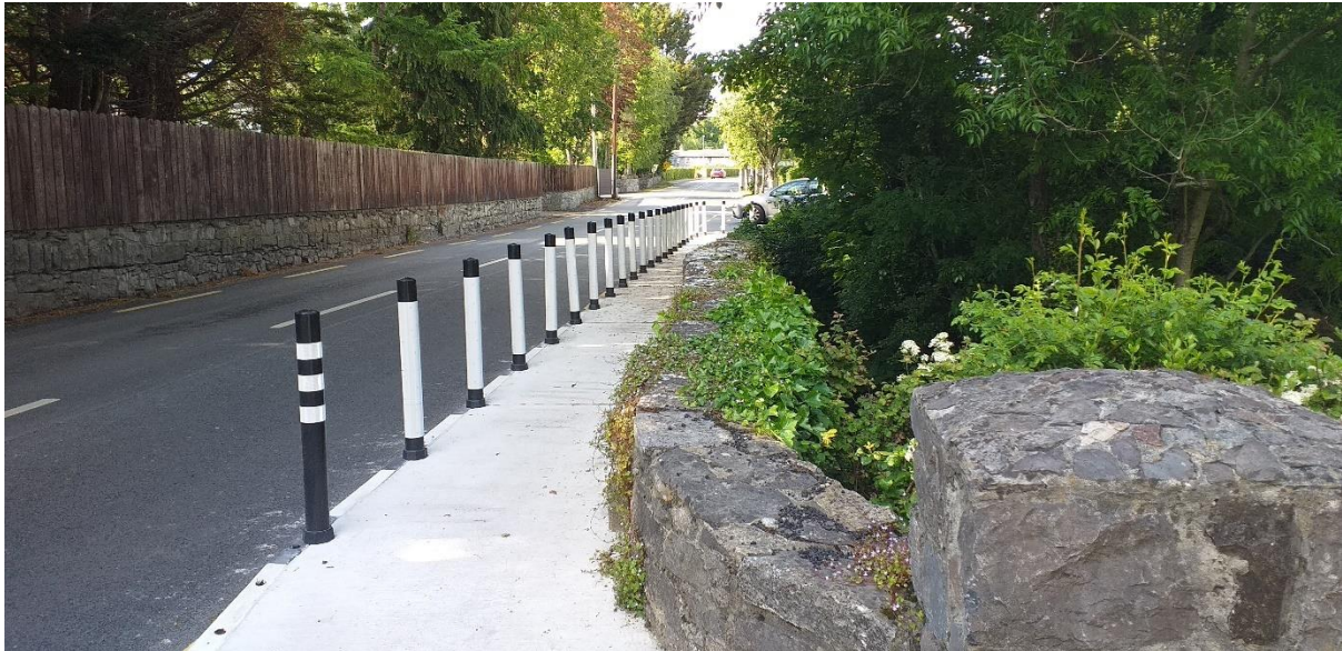
Existing Pausdeen Bridge with the temporary footpath and bollards looking towards Celbridge (to the North). See drawing 210303-03-123 for detail of the proposed works to the bridge
