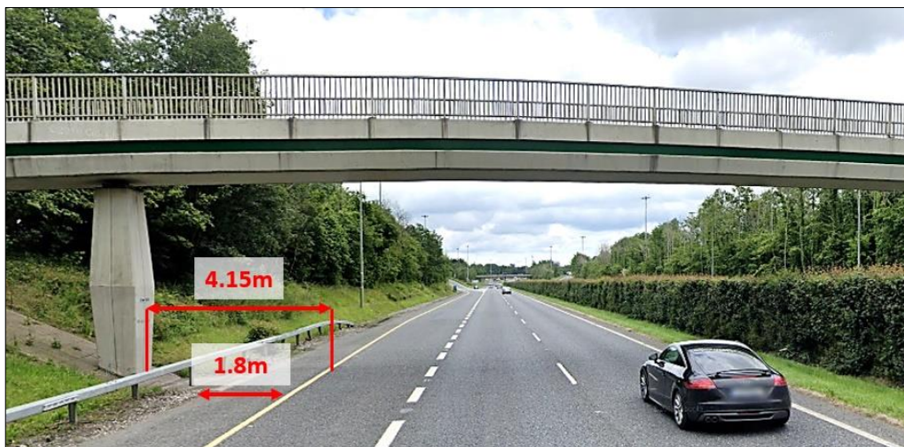
Figure 3.11: Cooldrinagh Lane Footbridge – Existing Offsets to adjacent Bridge Elements on Eastbound Carriageway (©2021 Google)
