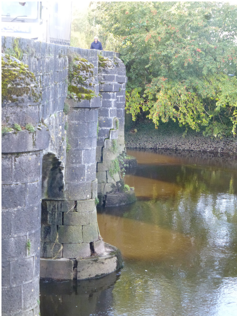
Fig 23. Scouring on the upstream side of the bridge has damaged the cutwaters and undermining pier dislodging masonry
