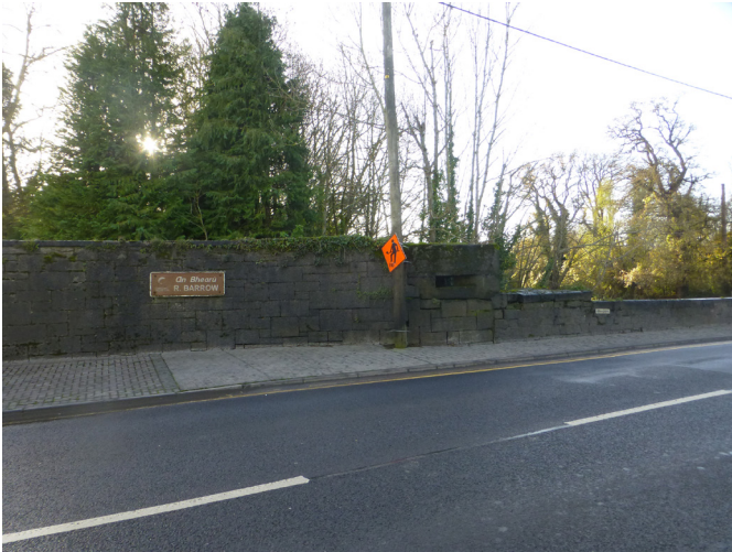
Fig 25. Displaced masonry with open joints
