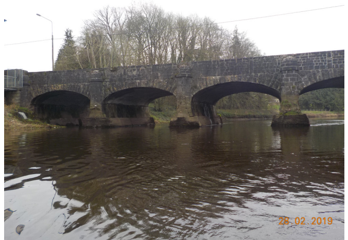
Fig 17. North side of bridge upstream - damage contributed to scouring at cutwaters
