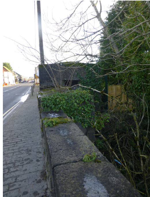
Fig 26. Localised rebuilding required to remove embedded roots
