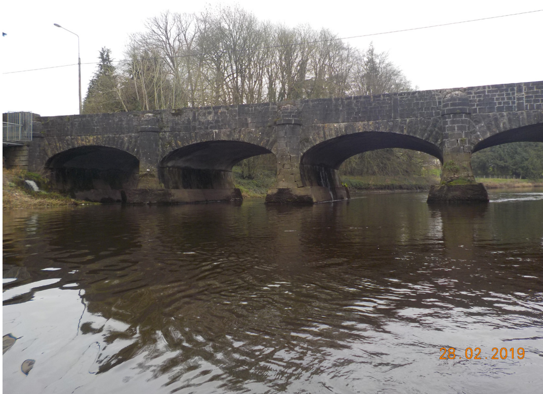
Fig 30. View to north upstream side of bridge , where settlement and displacement has occurred to pier structures
