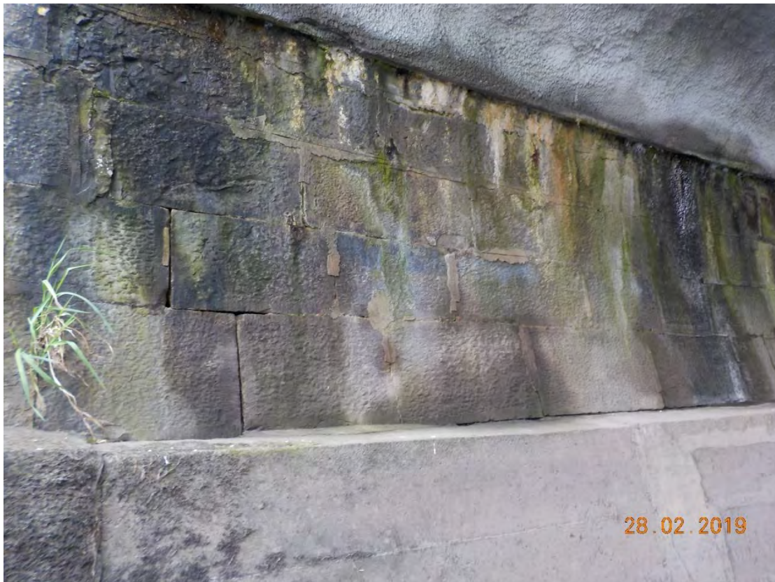
Figure 6: loss of mortar in joints and vegetation growth
