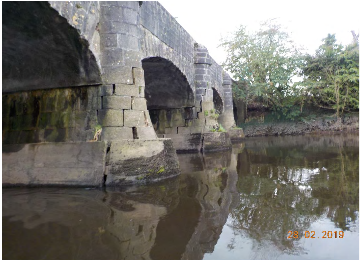
Figure 5: Cracking in concrete skirt and failure of masonry cutwater
