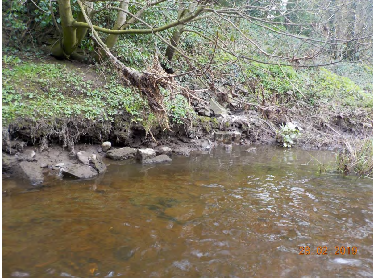
Figure 4: Scouring along downstream east embankment
