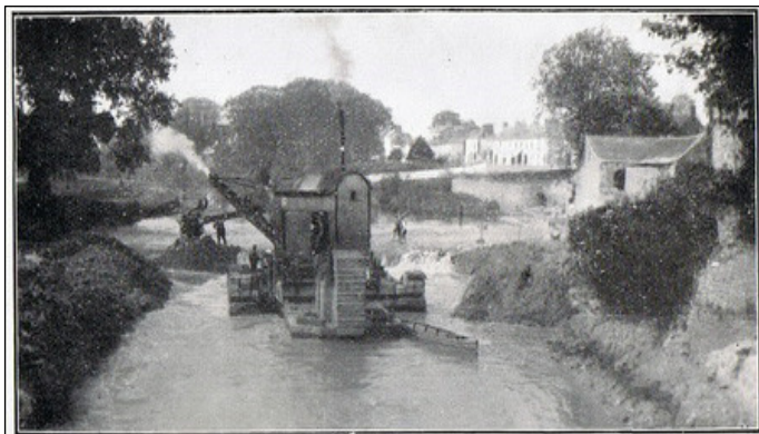
Plate 4 Dredging works at Monasterevin in the 1930s. This is the stretch of river immediately upstream of the subject bridge (Source: Irish Waterways History).
