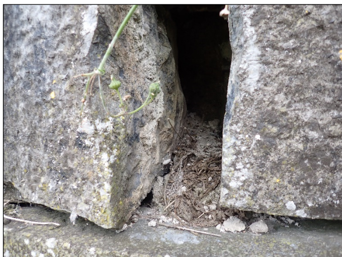
Plate 14 Large gaps present between stonework – evidence of old bird nests but these crevices are potentially accessible by rats and this will deter use by bats and birds.
