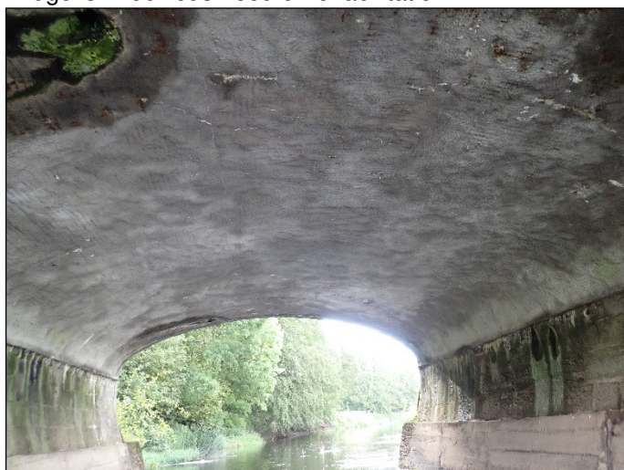
Plate 11 Evidence of previous maintenance works and filling of crevices at Monasterevin Bridge. This has reduced the potential for bats. The crevices present are in the shearwaters and generally low and large; such crevices are also potentially accessible by rats so bats less likely to use them.
