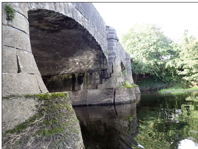
Plate 10 Upstream face of Monasterevin Bridge showing large cracks and spaces in the stonework. Bridge is in obvious need of rehabilitation.
