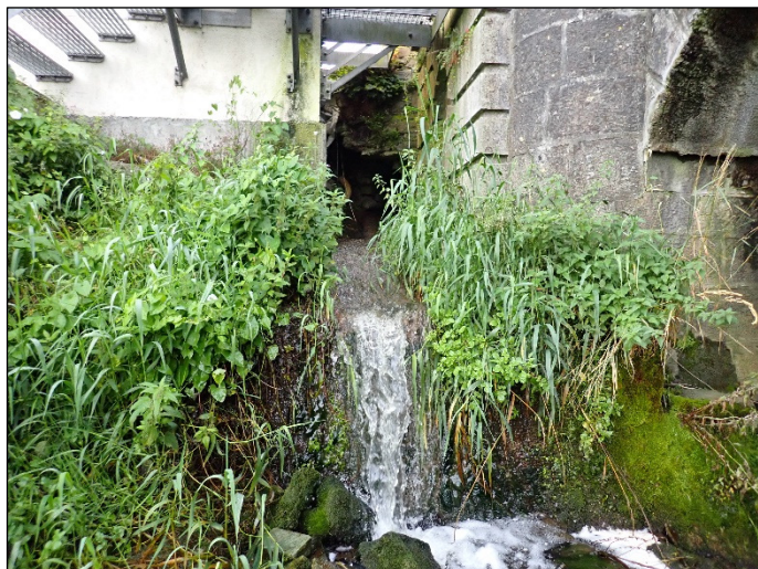
Plate 17 Discharge entering the River Barrow at the left bank beside the bridge.
