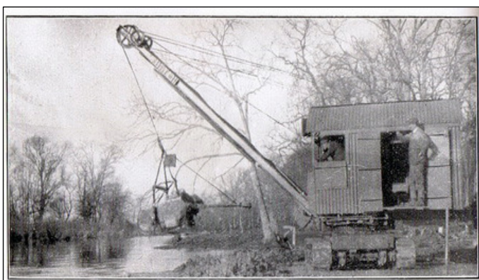
Plate 12 Dredging works at Monasterevin in the 1930s. The dredging works were undertaken using drag lines and the river was also diverted and dried out during the works. This scheme permanently altered the physical character the river (Source: Irish Waterways History).
