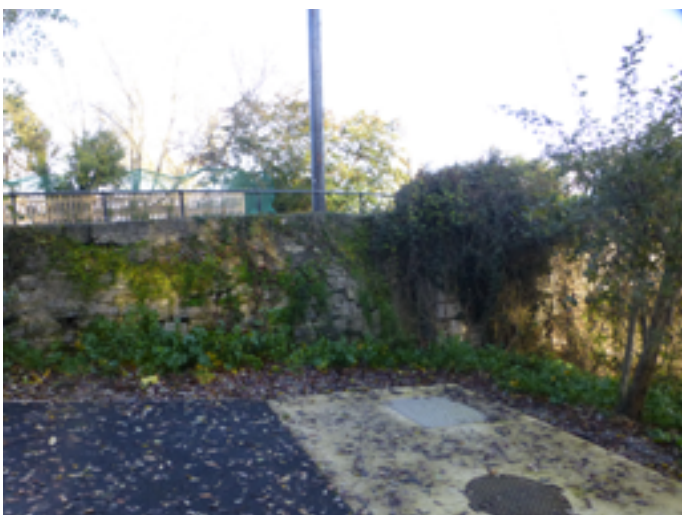
Fig 29. Repair to damage masonry required to west bank wing wall
