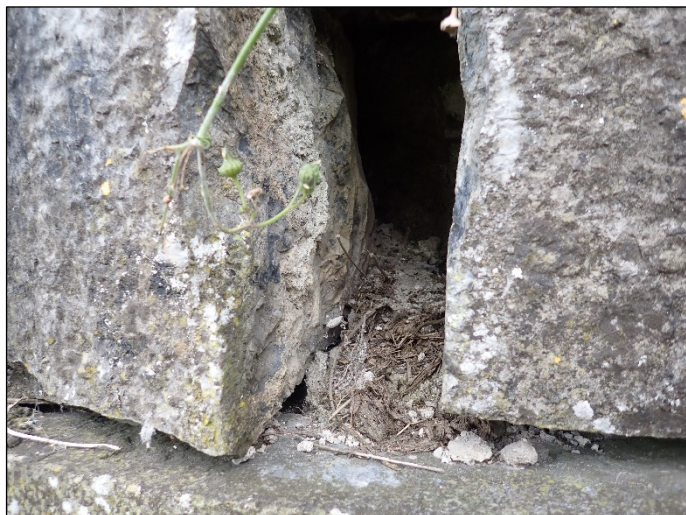
Plate 14 Large gaps present between stonework – evidence of old bird nests but these crevices are potentially accessible by rats and this will deter use by bats and birds.
