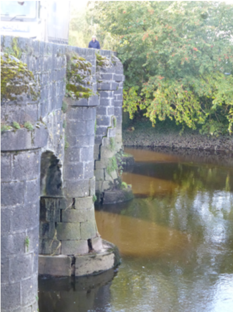
Fig 23. Scouring on the upstream side of the bridge has damaged the cutwaters and undermining pier dislodging masonry
