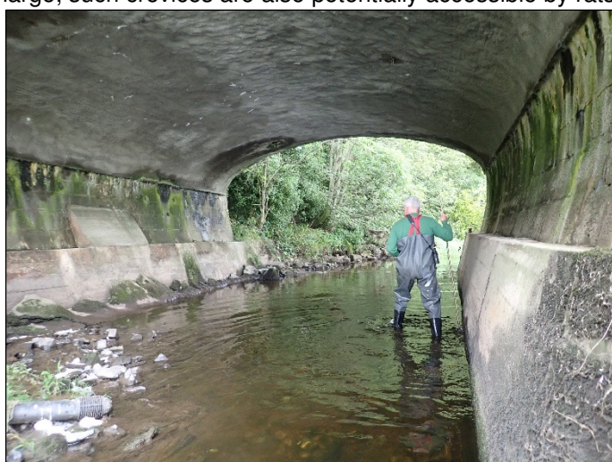
Plate 12 Left arch also showing previous filling / repointing. Only crevices at the top of the bridge are wet and seem to be receiving road runoff – making them unsuitable for use by bats.
