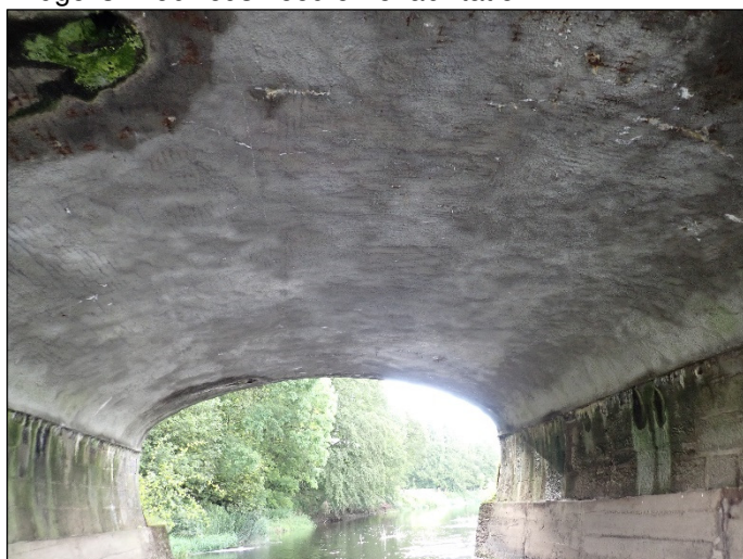
Plate 11 Evidence of previous maintenance works and filling of crevices at Monasterevin Bridge. This has reduced the potential for bats. The crevices present are in the shearwaters and generally low and large; such crevices are also potentially accessible by rats so bats less likely to use them.
