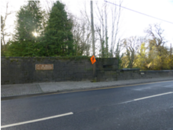
Fig 25. Displaced masonry with open joints
