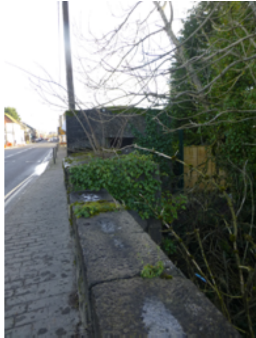
Fig 26. Localised rebuilding required to remove embedded roots
