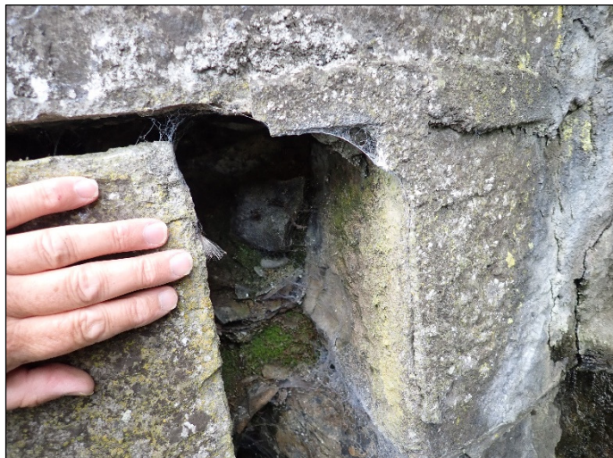
Plate 13 Large gaps present between stonework – but no evidence of bat usage was found.
