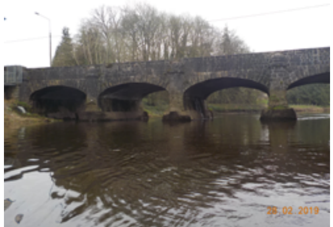
Fig 17. North side of bridge upstream - damage contributed to scouring at cutwaters
