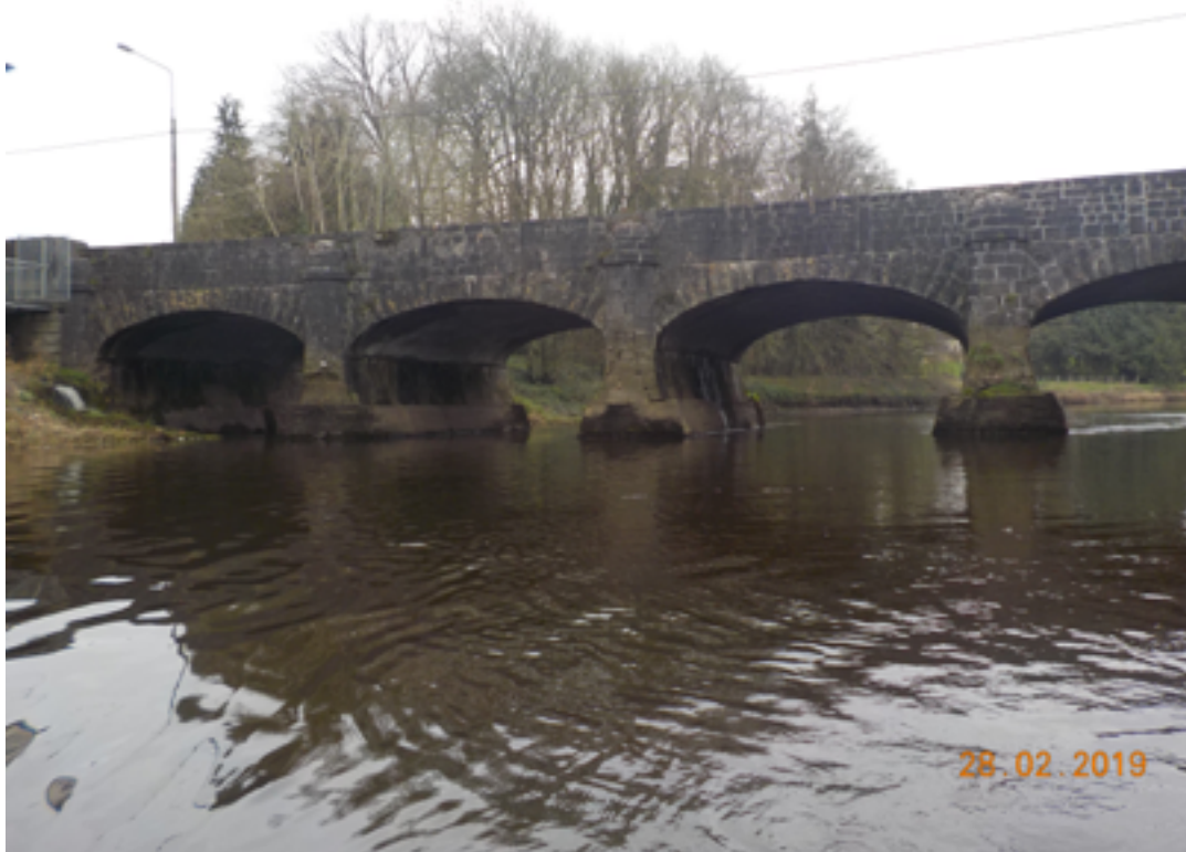
Fig 30. View to north upstream side of bridge , where settlement and displacement has occurred to pier structures
