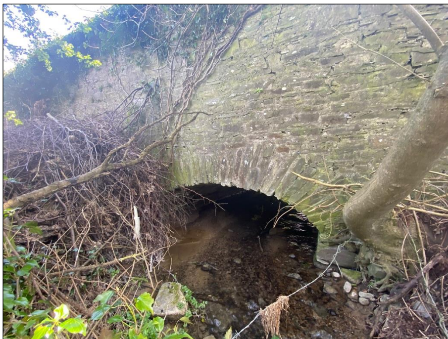
Plate 1 Moone Village bridge is very low with minimal space underneath, which is suboptimal for bats.
