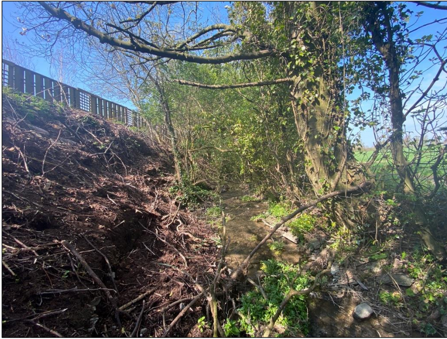
Plate 3 The upstream side showed clear evidence of recent vegetation clearance and debris.
