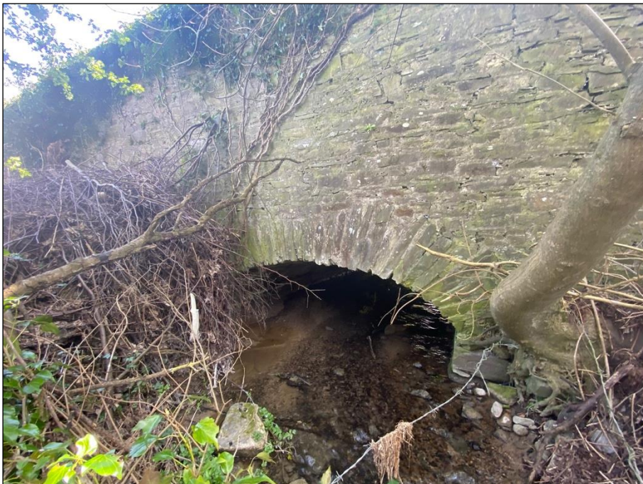
Plate 4 Moone Village bridge is very low with minimal space underneath.
