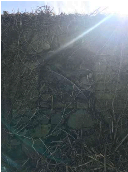
View of low level blocked archway
