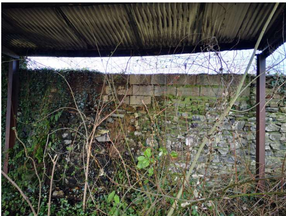
Later concrete blockwork wall intervention to historic stone wall of western ruins
