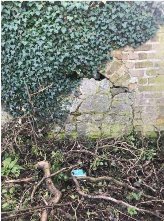
View of low arched opening
