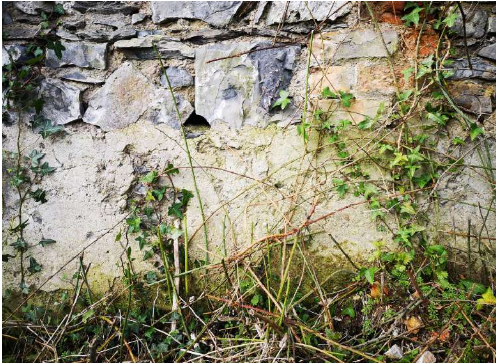
Remnants of lime render to base of wall
