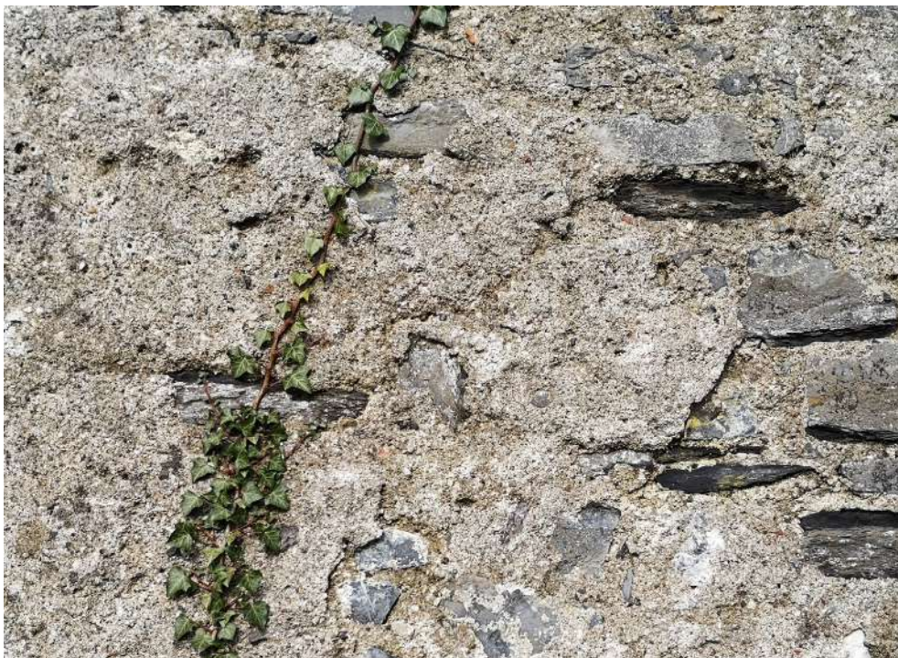
Remains of lime render to gable wall
