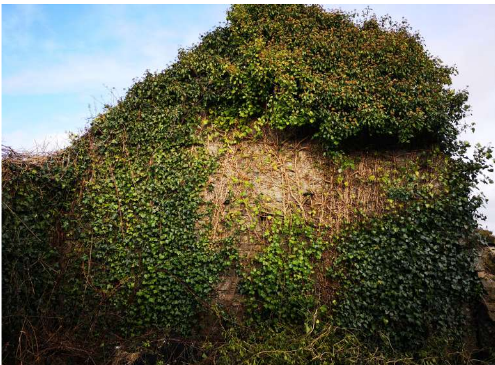
View of southern gable wall with overgrowth
