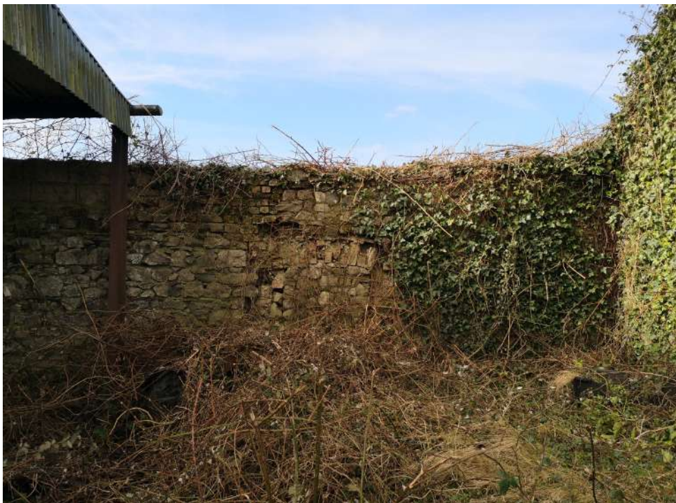
View from agricultural shed to Southern gable of North-Western ruin - extensive overgrowth has limited access to this gable elevation
