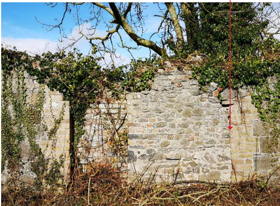
Detail of original blocked 2.8m opening to centre of southern stone wall
