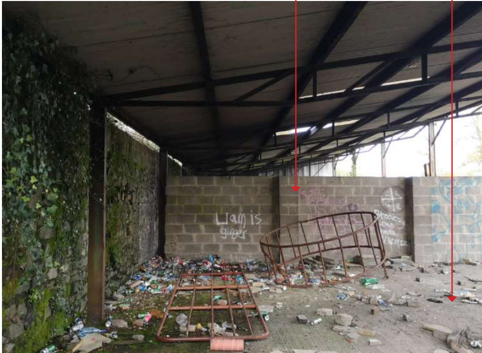
View of mono-pitch roof and steel structural supports to Western stone wall
