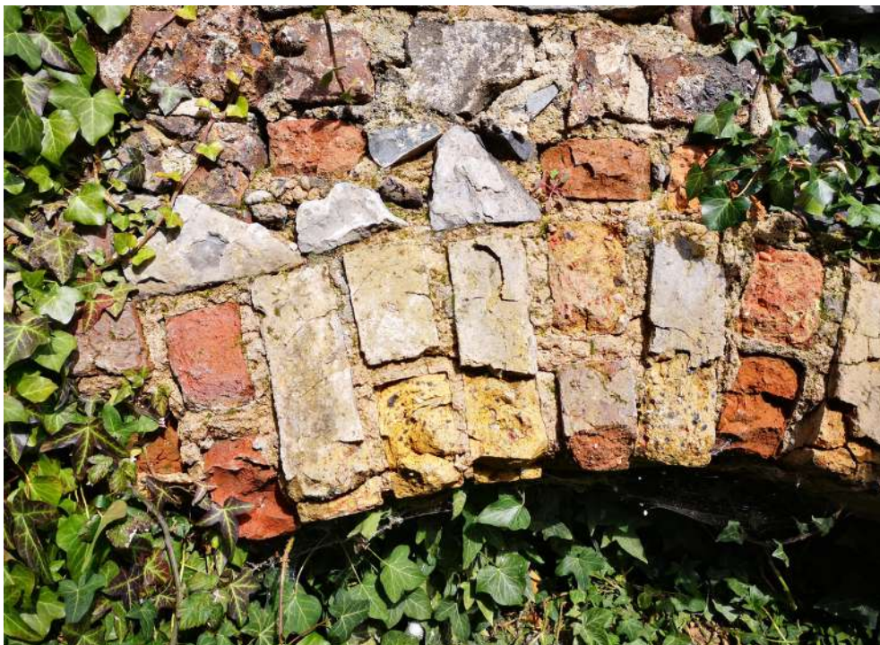
Delamination of brickwork evident at archway to window opening
