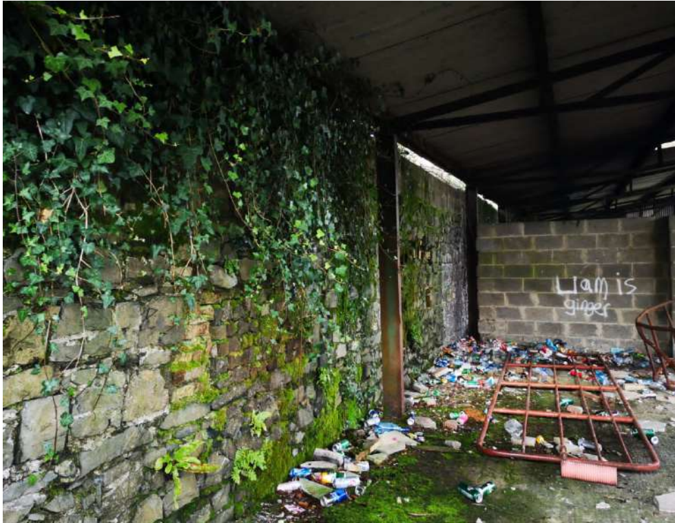
Water penetration damage and overgrowth apparent to Westen stone wall
