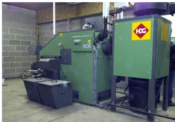
Figure 12.0 Biomass Boiler and Fuel Hopper
