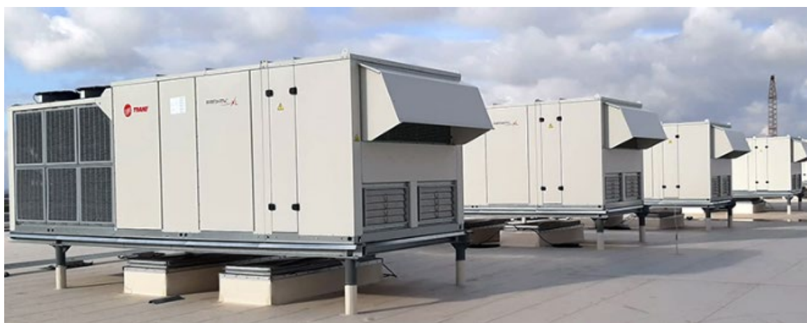
Figure 3.0 Typical Rooftop Heatpump Unit
