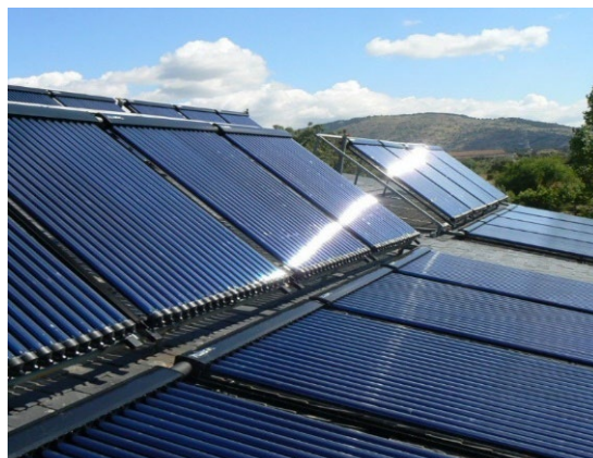
Figure 11.0 Roof Mounted Solar Water Heater
