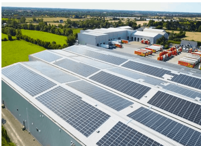
Figure 8.0 Roof Top Commercial Solar Photovoltaics Panels
