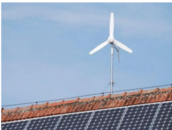
Figure 9.0 Roof Mounted Wind Turbine
