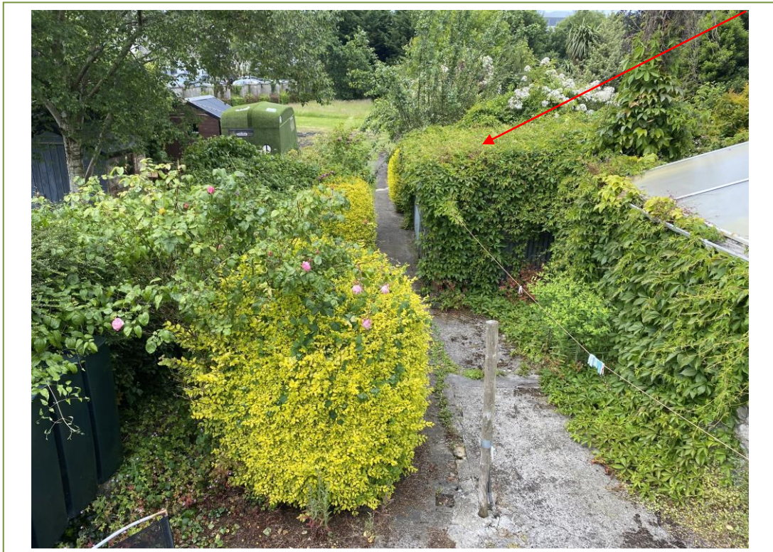
The garage roof is currently overgrown
