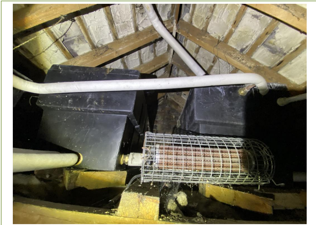
Plastic water tanks
