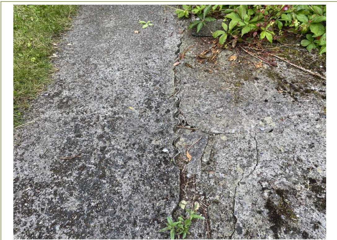
Small area of cement sheeting concreted into the ground
