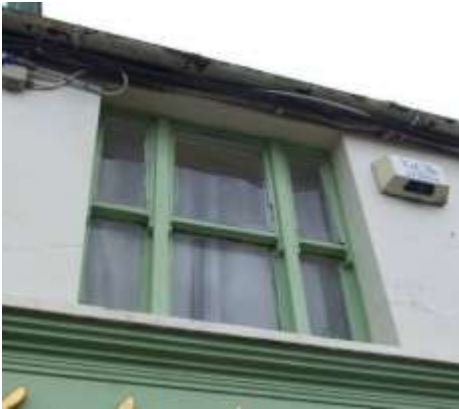
Fig. 105: Historic windows are perhaps the single most important element of an historic streetscape
