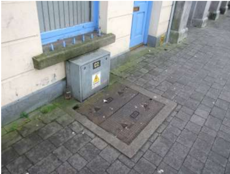
Fig. 116: Poor consideration in the location of service boxes
