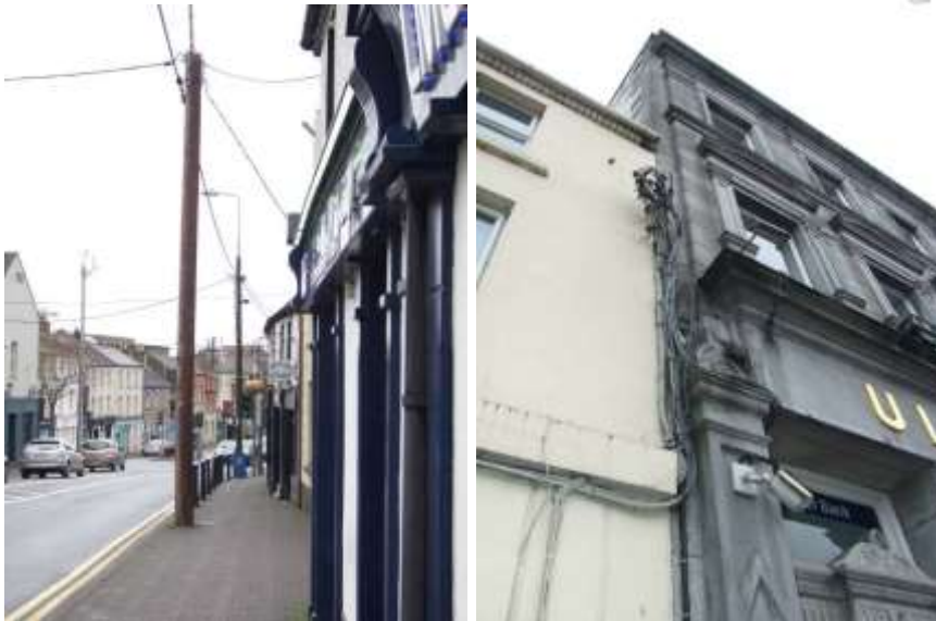
Fig. 124: Proliferation of masts and cables in street spaces (left) and redundant fittings on elevations (right)
